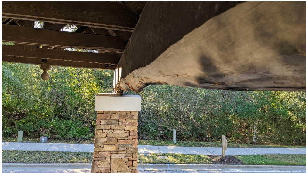
Photograph No.2 – Damaged wood beam at interior surface.
