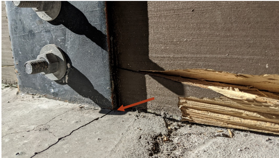
Photograph No.4 – Splitting at the column side beam connection
