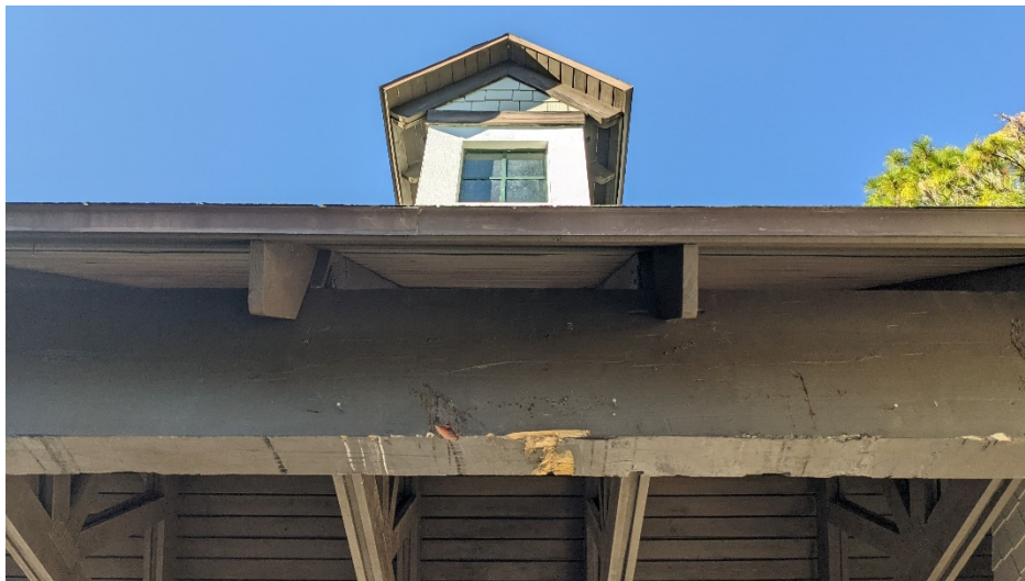
Photograph No.6 – Minor surface damage at the exit of the ranger station
