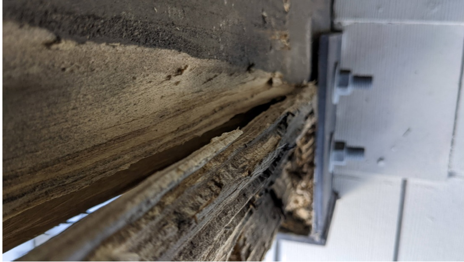
Photograph No.3 – Splitting at the building side beam connection
